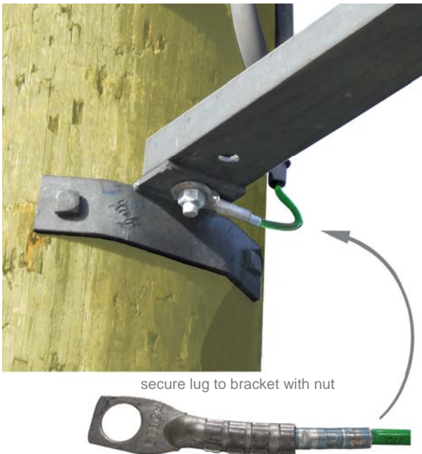
Figure 3.3c, Routing Ground Wire
